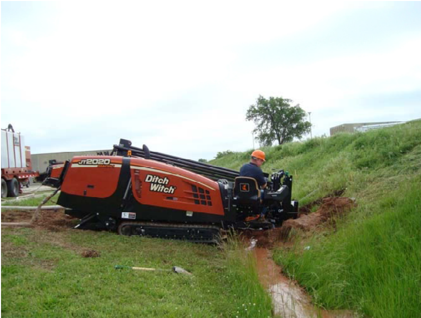
Figure 1. Drilling horizontal borehole into embankment as done for borehole #1. (Operator Blaine Easter, Charles Machine Works, Inc.)
