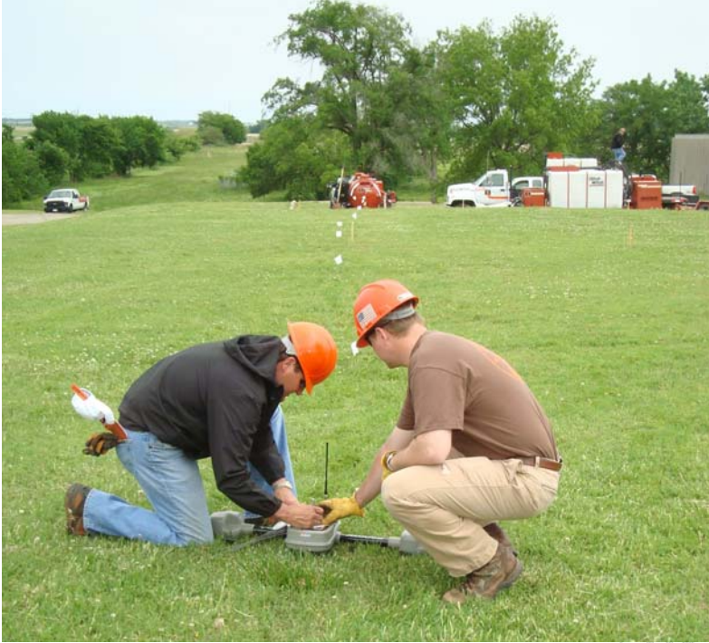
Figure 3. Operators recording location of beacon on drill pipe. (Gary Lawson, left, and John Lamerton, right, Charles Machine Works, Inc.)
