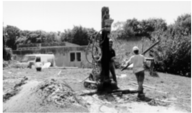
Workers drill the holes for the ground heat exchanger at Charlestown J&I School.
